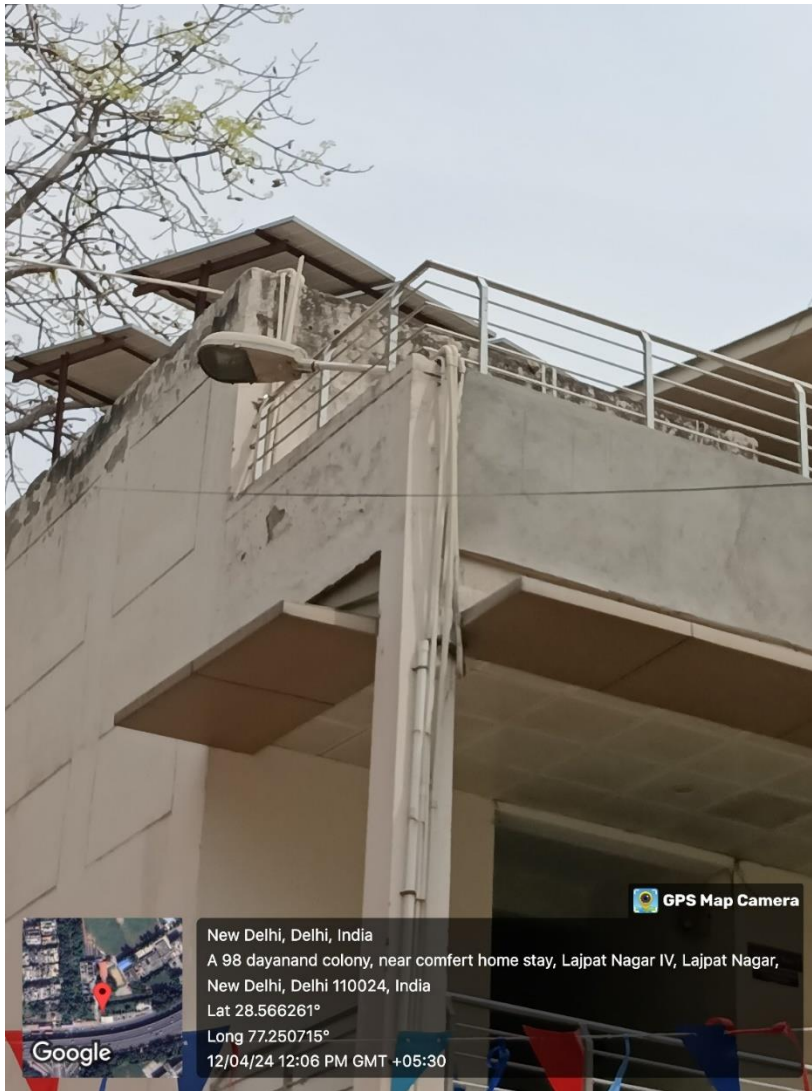
Fig III. 3 : Solar panels at rooftop of PGDAV college
